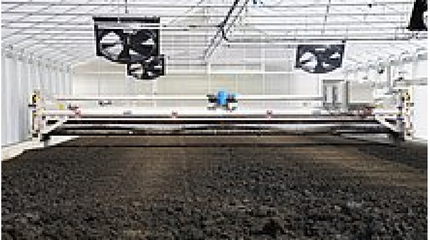
The HUBER Sludge Turner SOLSTICE® makes solar drying a success
