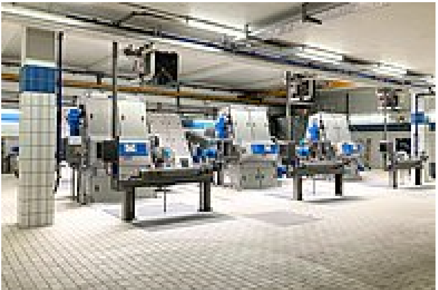
The "anniversary machine" RakeMax® in its basic version in the main inlet of a wastewater treatment plant.
