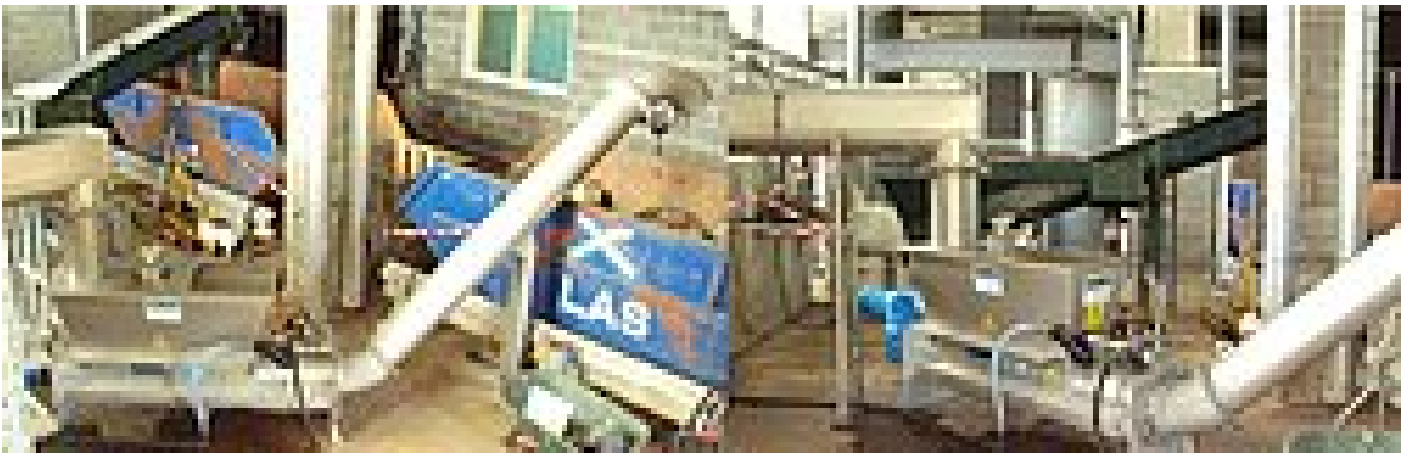
New WAP/L BG4 Screenings Handling Unit
