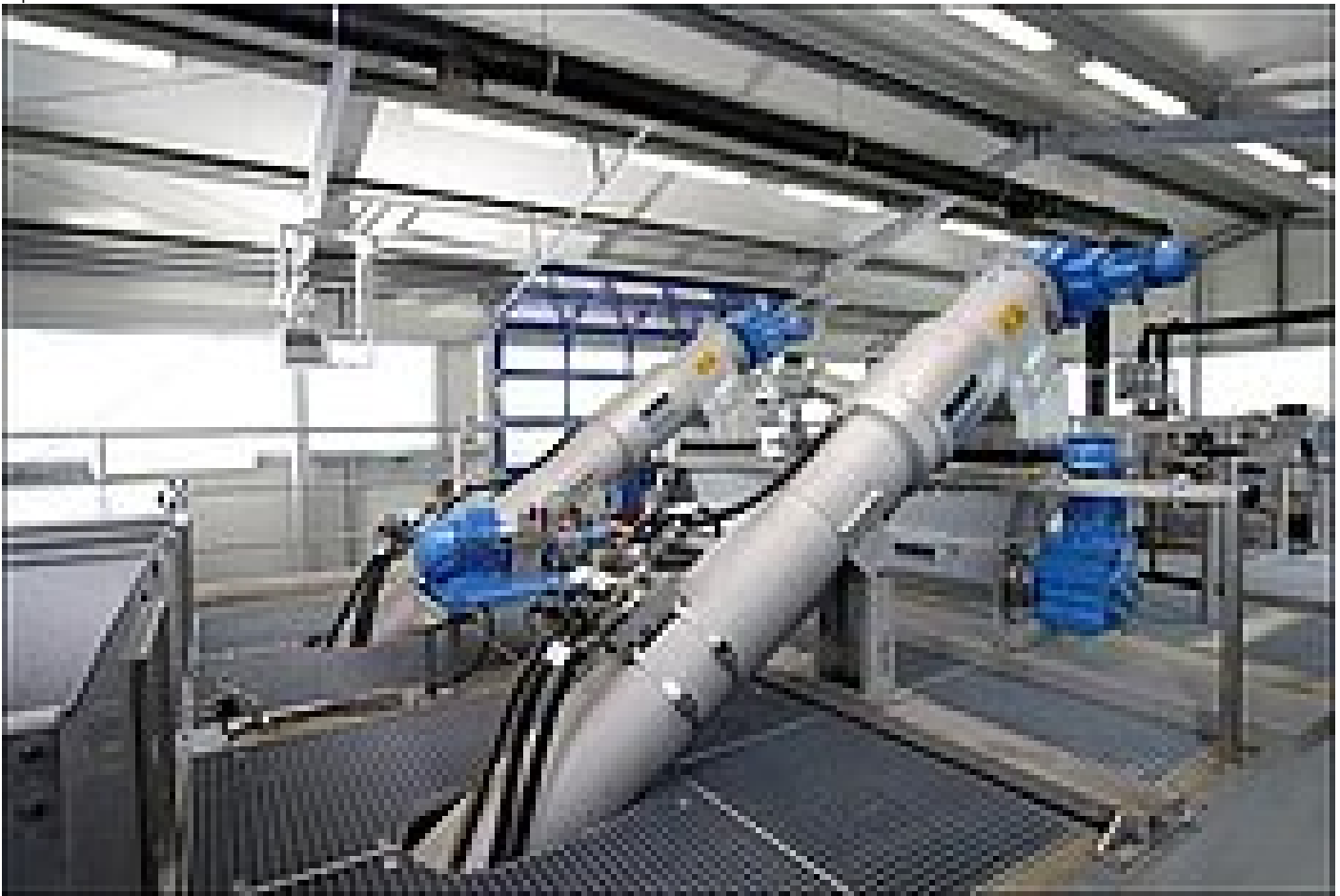
The coarse screen is a 5 mm STEP SCREEN®, the fine screen is equipped with a 1.0 mm mesh. The screenings from the fine screen are dewatered and discharged into a container
