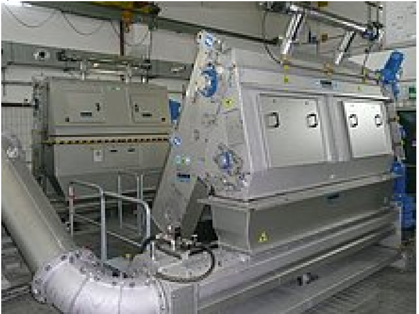
Back view of line 1
