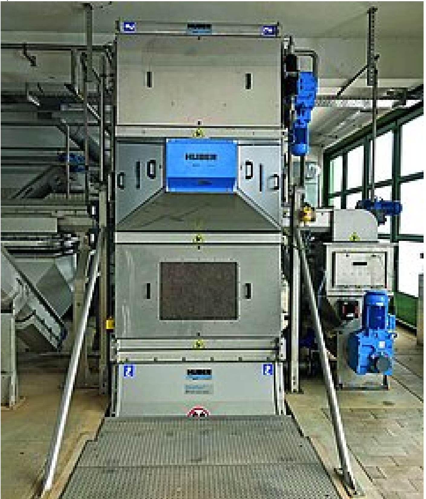
"Safety Vision" installation, running to the full satisfaction of the plant operators
