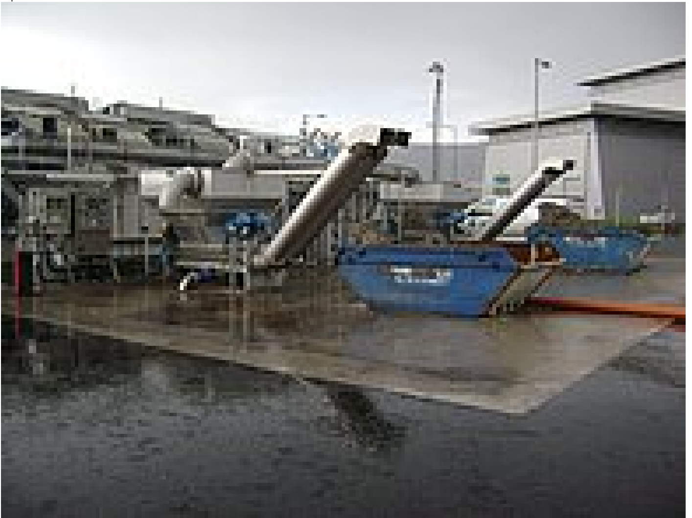
2 off HUBER Wash Press WAP-SL units designed for 15 m 3 /h raw screenings, via launder channel
