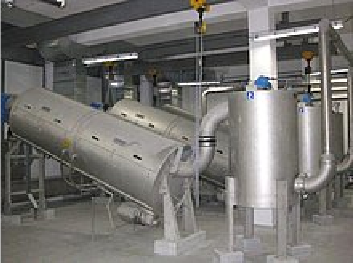
Three ROTAMAT@ Screw Thickeners RoS 2 with upstream flocculation reactors
