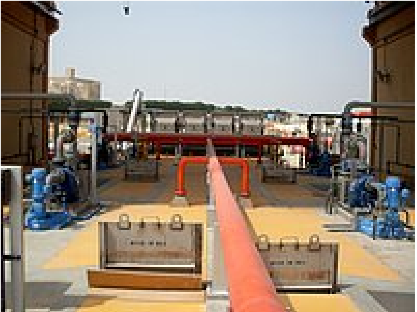
Installation with a set of 4 VORMAX units
