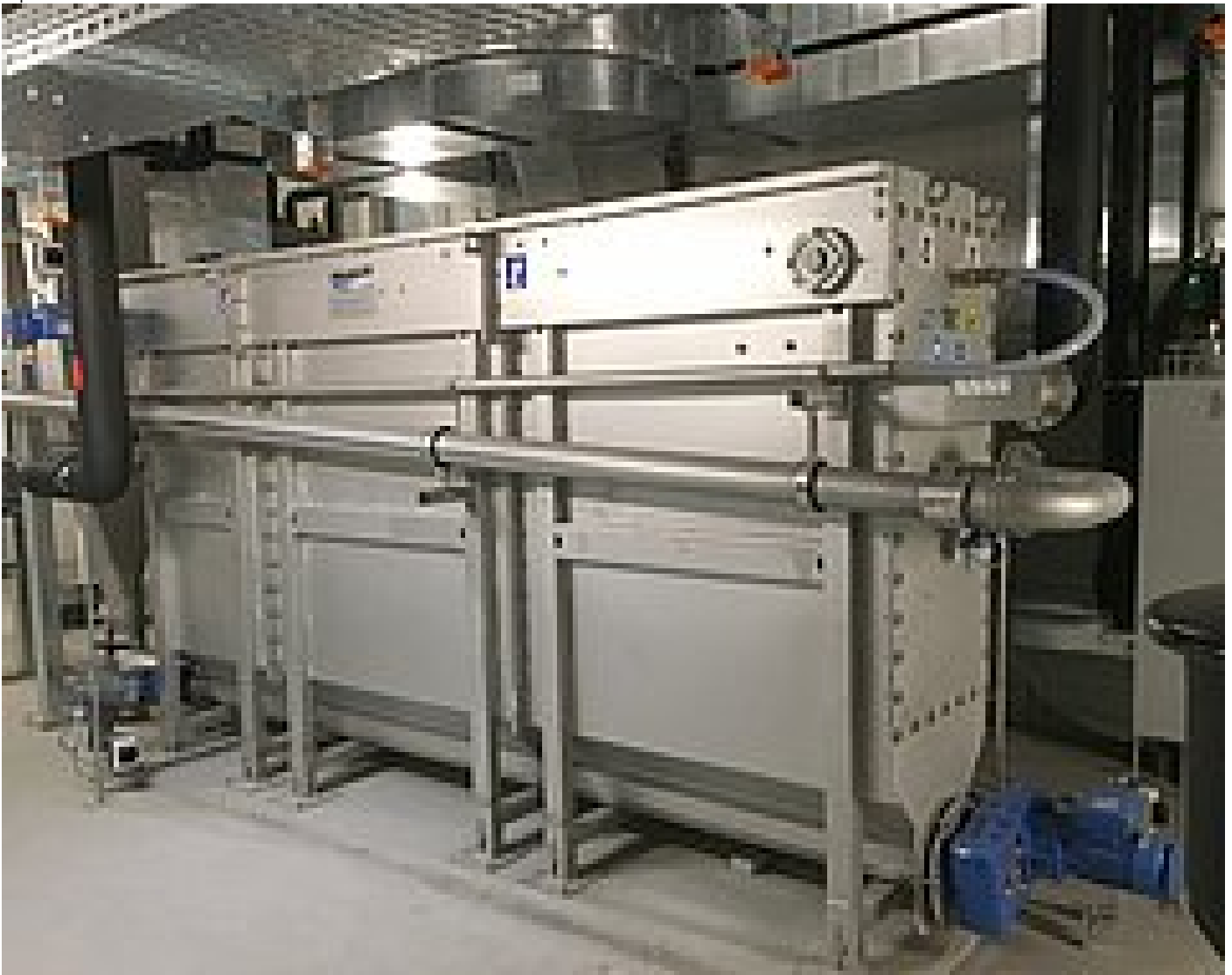
Fig. 3: HUBER Heat Exchanger RoWin in the technical equipment room of the Valsana hotel
