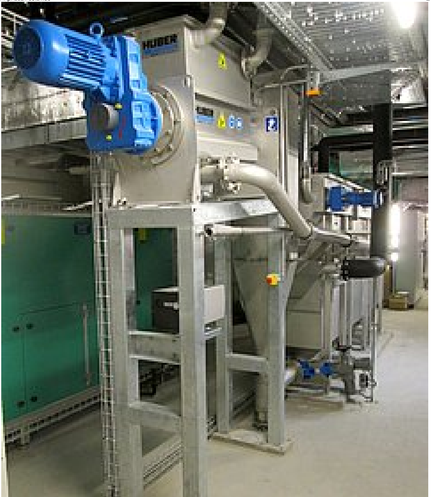
Fig. 2: Pre-screening (6 mm) of wastewater with HUBER Wash Press WAP®
