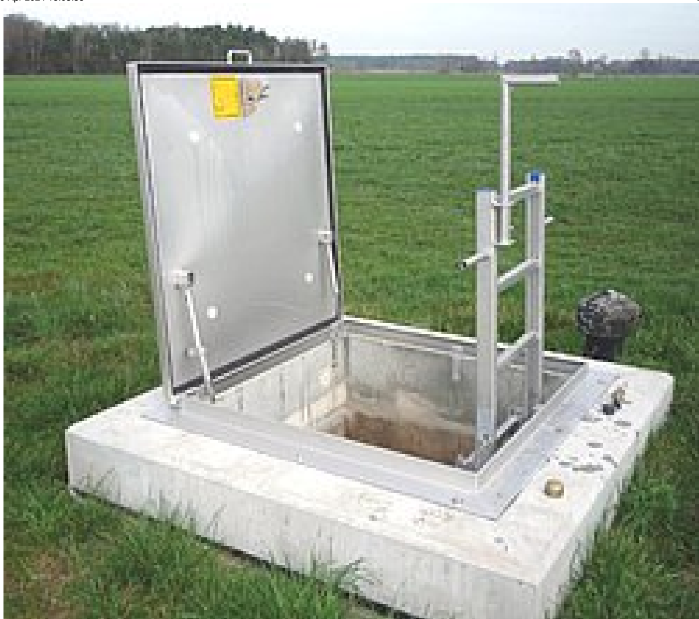
Safe equipment: manhole covers, safety access ladder and entrance aid
