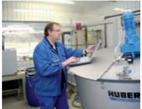
HUBER maintenance service
