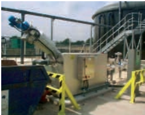
Outdoor installation of a Sludge Acceptance Plant for sludge screening
