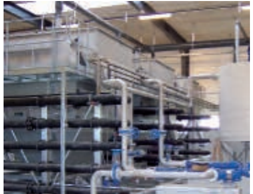
HUBER Dissolved Air Flotation Plant HDF with chemical treatment stage
