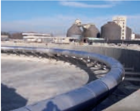
HUBER Submerged Effluent Pipes – optimal flow pattern below the water surface
