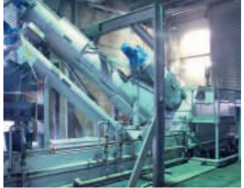
HUBER ROTAMAT® Complete Plant Ro5 BIO installed at an organic waste fermentation plant
