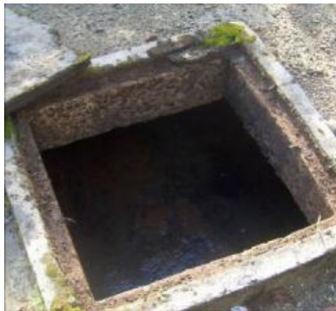
Septic Tank in Indonesia
