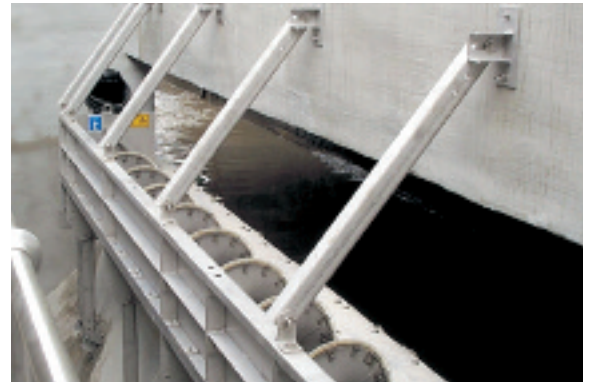
Attached with brackets to an inclined overflow weir
