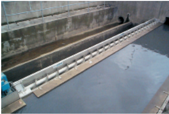
Bolted to a vertical concrete weir of a combined sewer overflow structure
