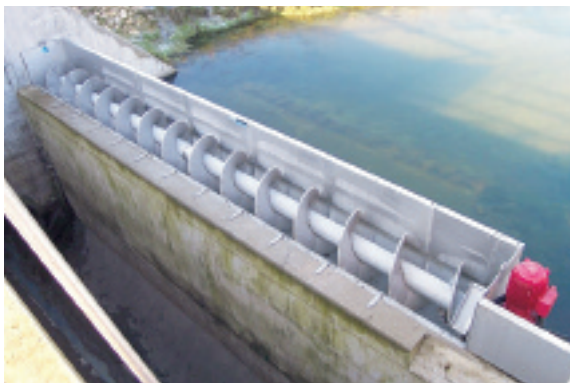
Installation at the overflow of a storm water retention basin
