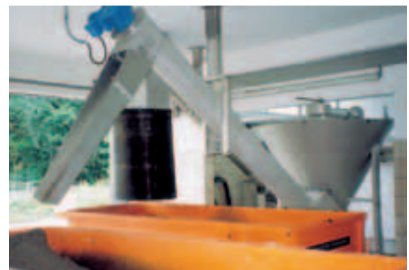
COANDA Grit Classifier discharging into a dumpster
